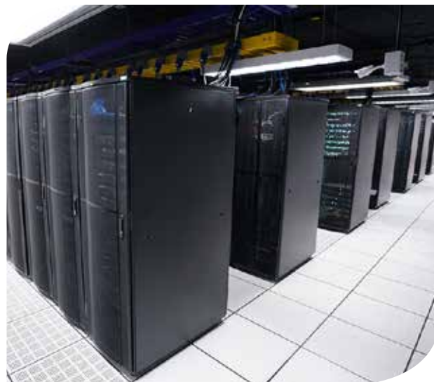
PROEN Internet Data Center (IDC)
